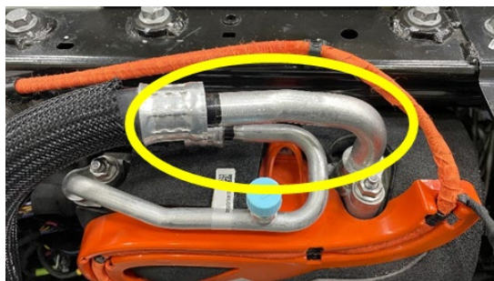
Figure 1- Foam Not Installed (China)
