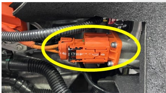
Figure 5 – Cover Not Installed
