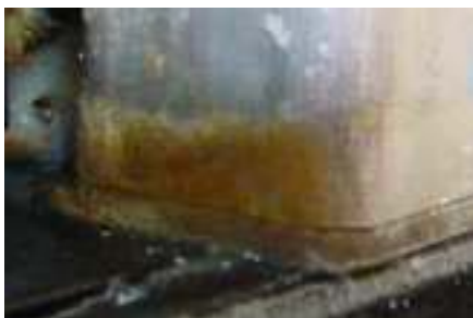
Figure 2 (Discoloration due to electrolyte leakage)
