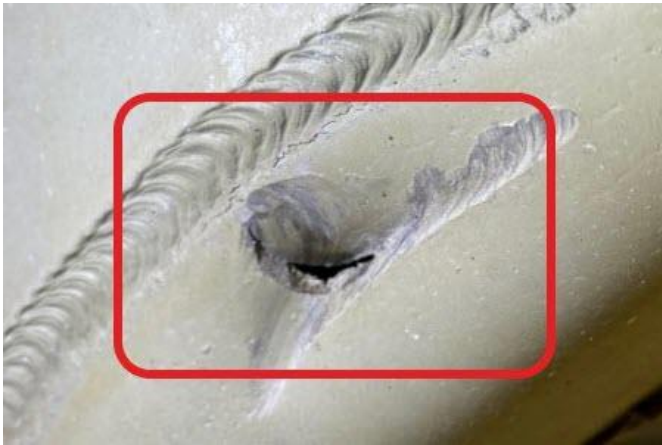
Figure 1 – Visible open hole
