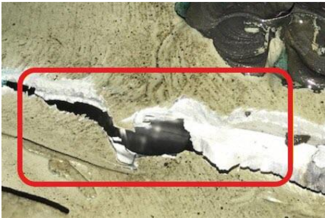
Figure 3 – Visible open crack
