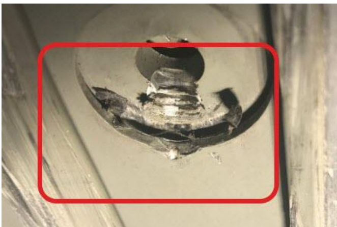
Figure 5 – Visible open crack
