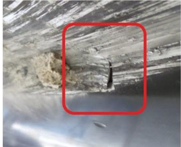
Figure 2 – Visible open crack
