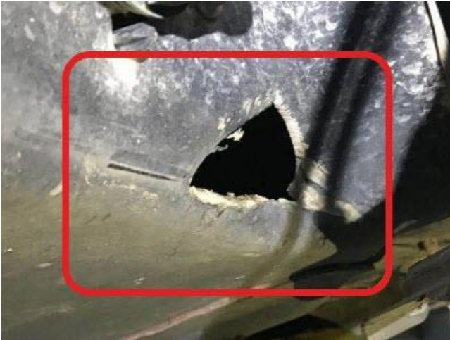
Figure 1 – Visible open hole
