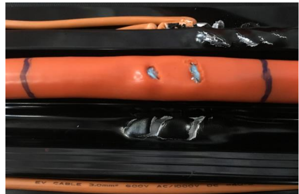
Figure 17 – Damaged cable under center ski
