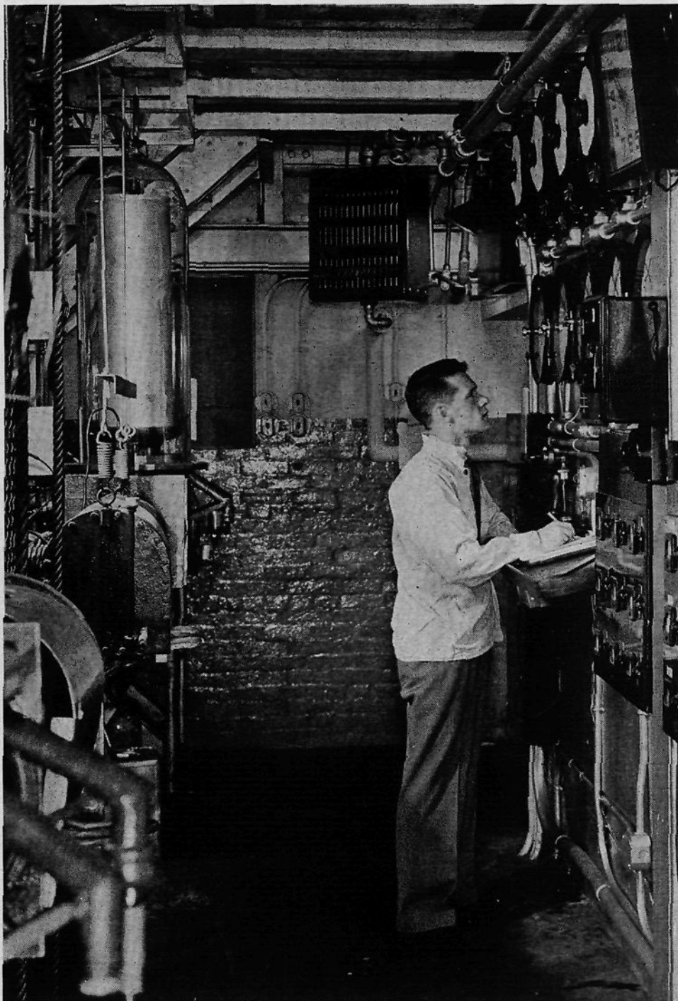
FIG. 9. Industrial falling-film still. Glass dome on the left covers the fifth evaporator in a succession of individual stills. The panels for controlling temperature and pressure are shown on the right.
