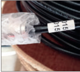
Fig. 17: Three 50m coaxial cables M&P Ultraflex7 well stored and labelled
