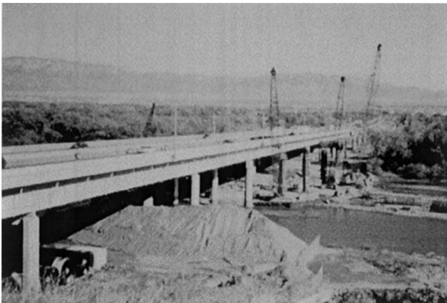
Figure 13. I-40 bridge over Rio Grande in Albuquerque, NM, U.S.A. (courtesy of Los Alamos National Laboratory).
