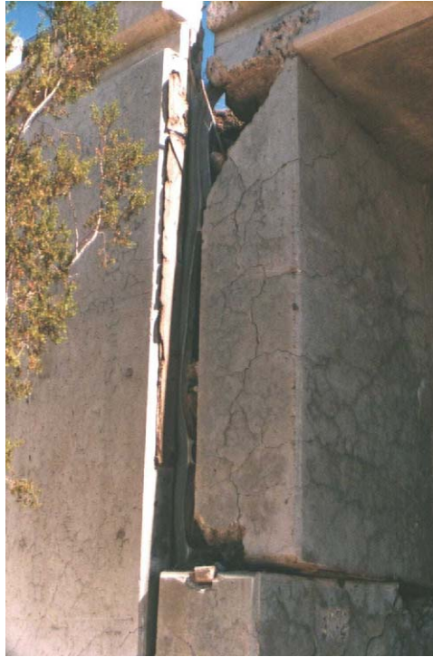
Fig. 6. Damage and misalignment of east wingwall and pier at south bridge abutment.
