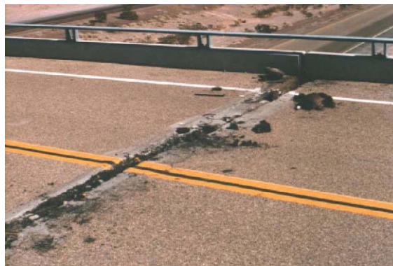
Fig. 5. View of damage to south abutment expansion joint.
