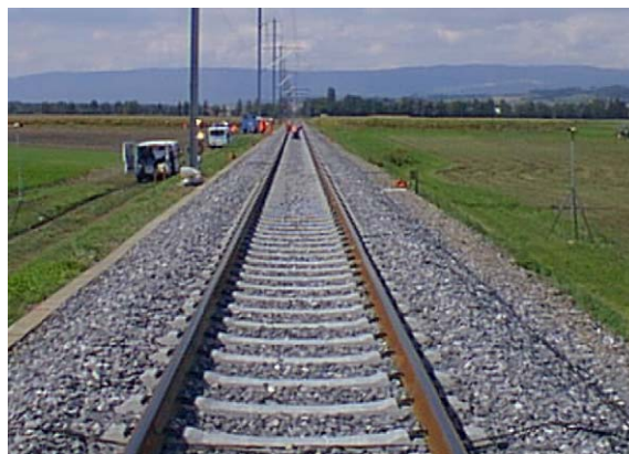
Fig. 1. Picture of the track section near Kerzers, where the measurements were performed.
