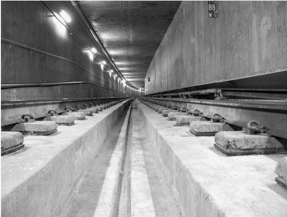
Fig. 8. Photograph of resiliently supported half-ties (LVT track) in the San Francisco Airport Extension subway.
