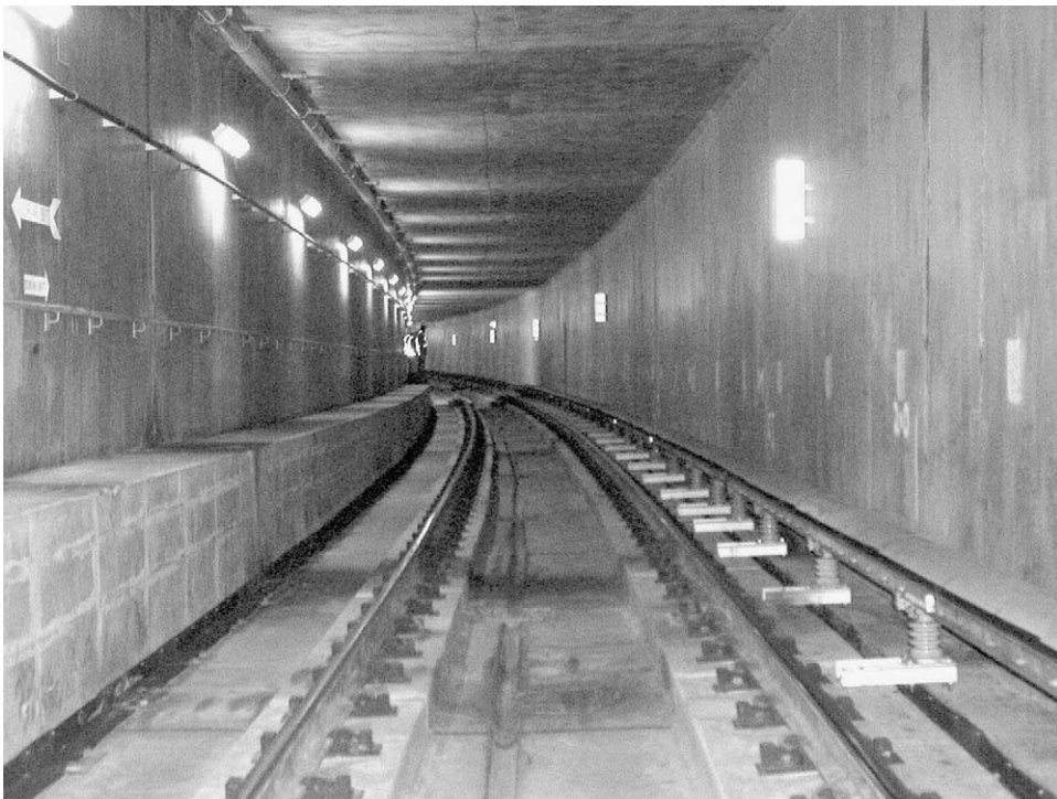
Fig. 9. Photograph of continuous floating slab track section in the San Francisco Airport Extension subway. Because there are no gaps between the floating slab and the subway invert larger than a few inches, impact testing from the invert to the surface was not feasible for this section of track.
