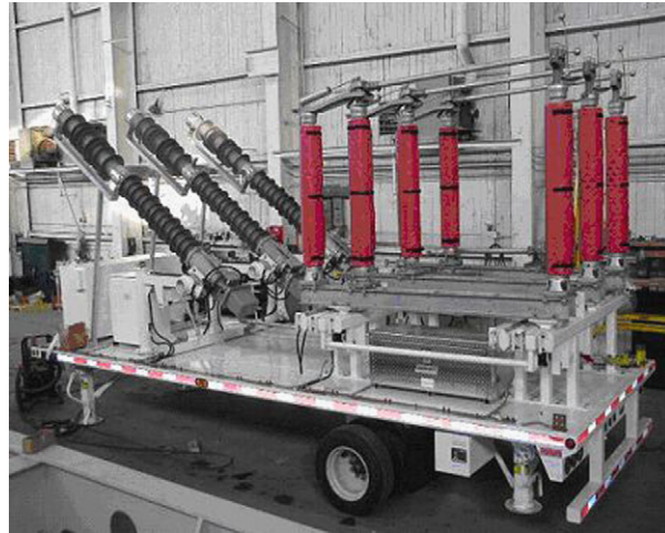
Fig. 1. A mobile substation.
