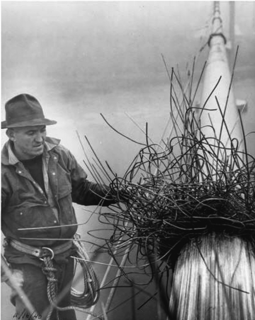
Fig. 5. Broken cable wires at north midspan cable band (from Ref. [9], with permission from Washington State Department of Transportation).
