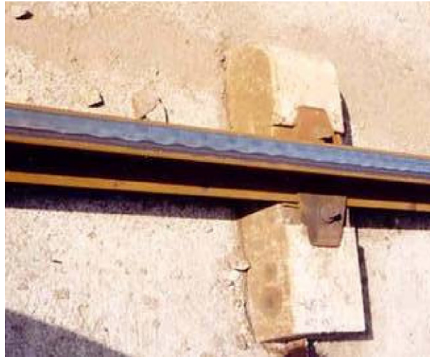
Fig. 1. Corrugation observed on the rail.
