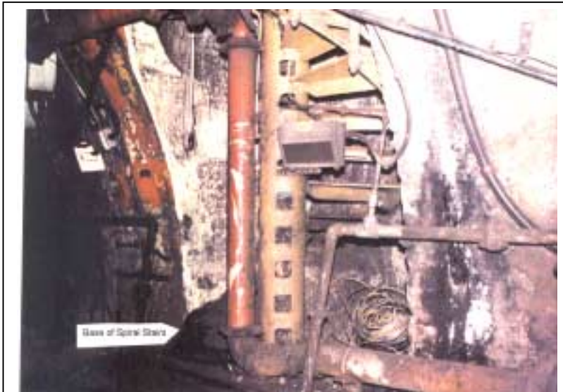
A narrow 10 flight spiral staircase serves as an evacuation route for passengers as well as a means for rescue workers to enter the tunnels.
