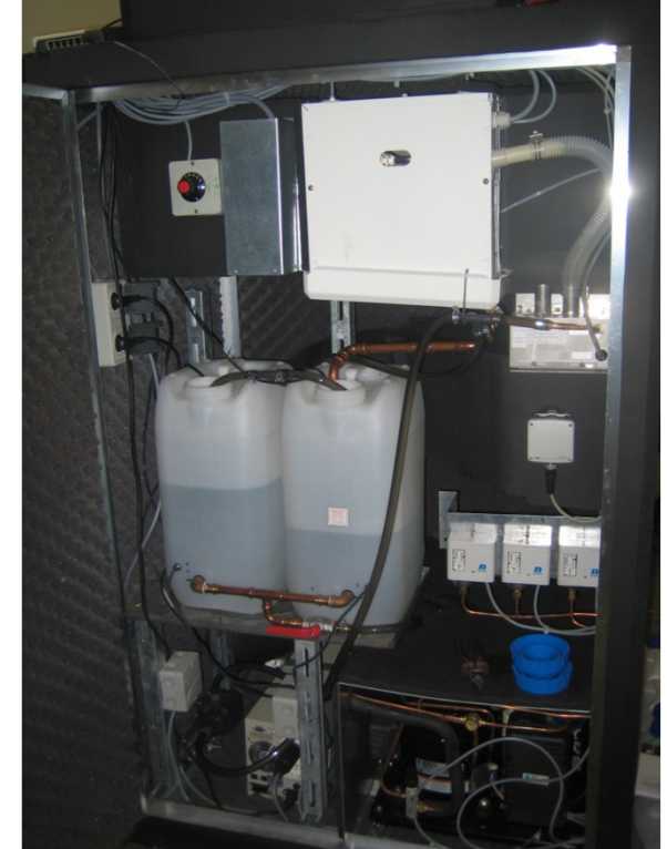
HVAC: separated from chamber for vibration isolation
